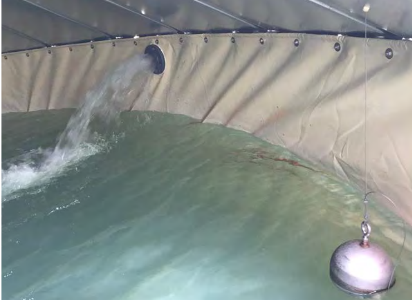
The type of liner chosen for the interior of a water storage tank is critical. It will determine water quality and needs to meet any requirements set by local governments or certification agencies.
